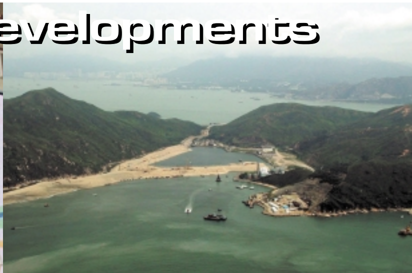
The site of the future Hong Kong Disneyland at Penny's Bay, Lantau Island. Reclamation work is now in progress and the opening of the Disneyland-style theme park is targeted for 2005/2006
